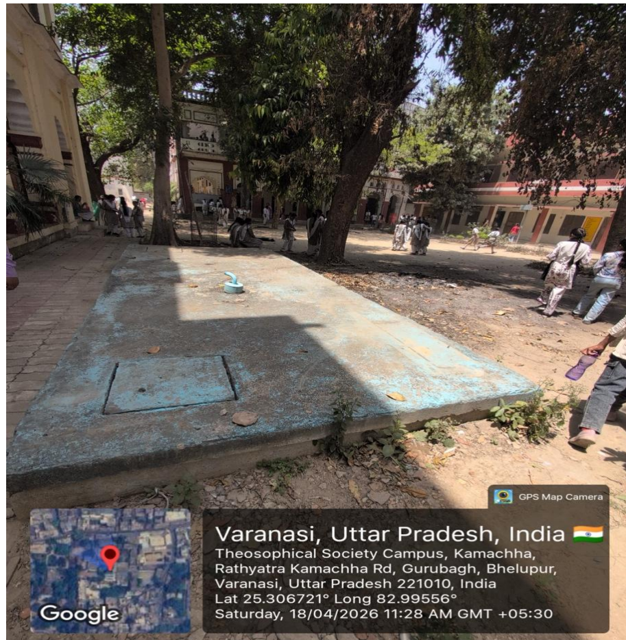
Fig. 4 Rainwater harvesting infrastructure installed on the college premises.
