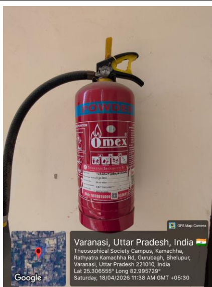
Fig. 9 ABC-MAP 90 type Fire Extinguisher installed at each floor of the campus building.
