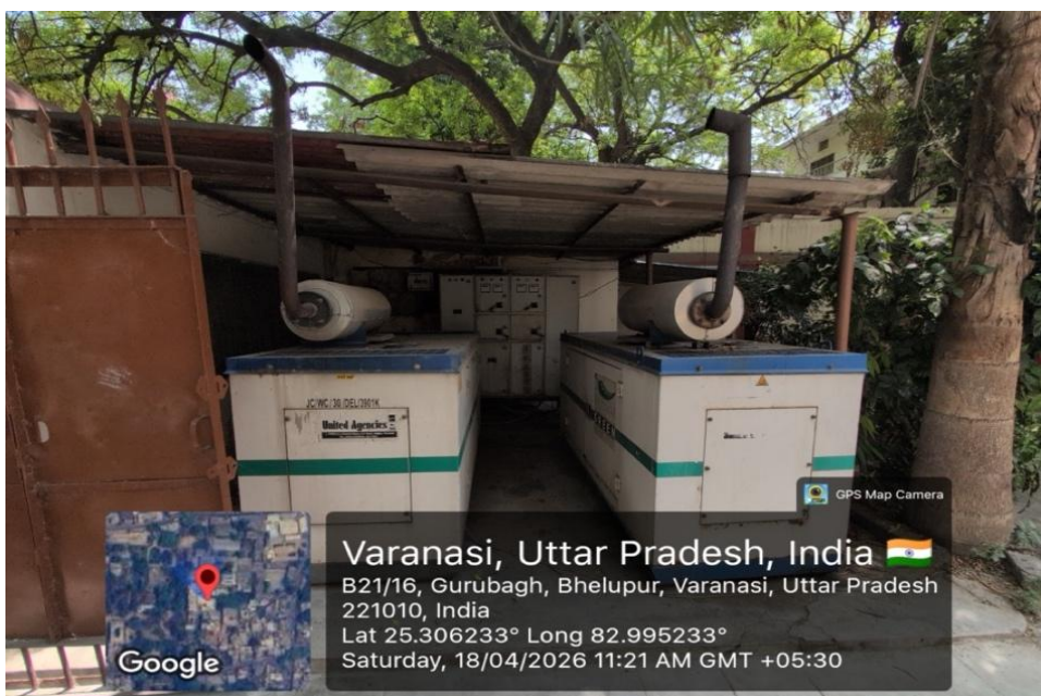
Fig. 6 DG sets installed for electricity backup on the college campus.
