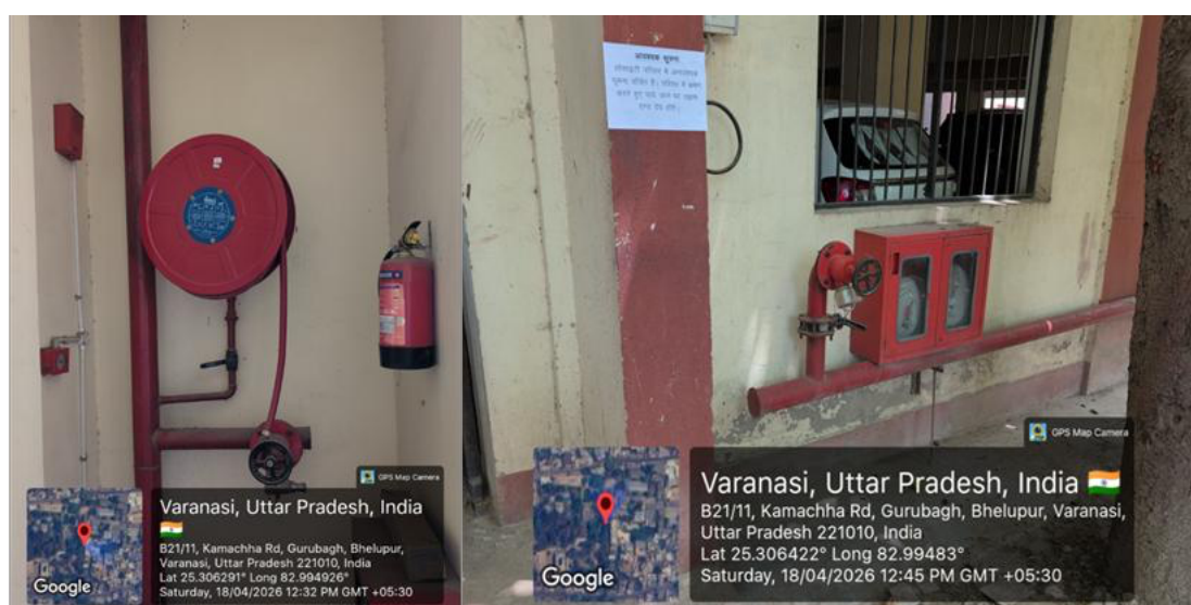
Fig. 10 Fire Fighting System installed in Leela Sharma Block of VKM.
