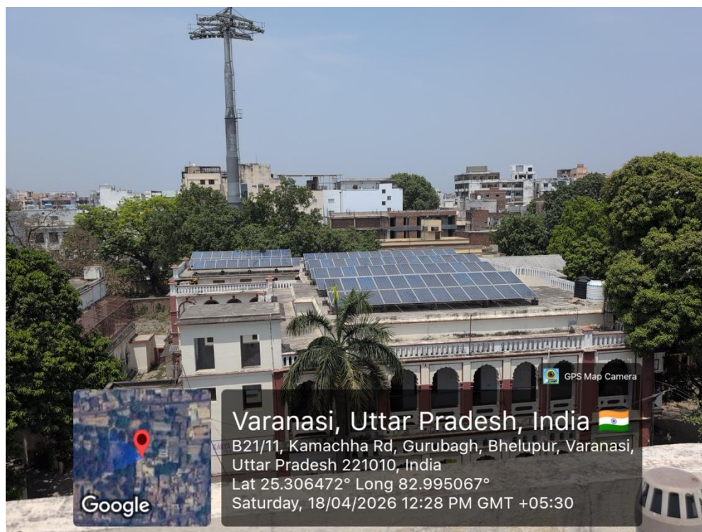
Fig. 7 Rooftop Solar Panels installed for renewable energy generation on the college premises.
